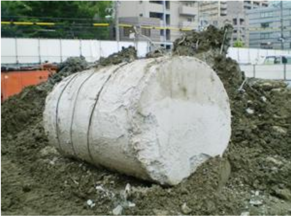
Underground obstacle removal situation (underground beam) (地中障害物撤去状況-地中梁)
