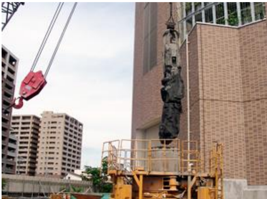
Underground obstacle removal situation(cast-in-place pile) (地中障害物撤去状況-場所打ち杭)
