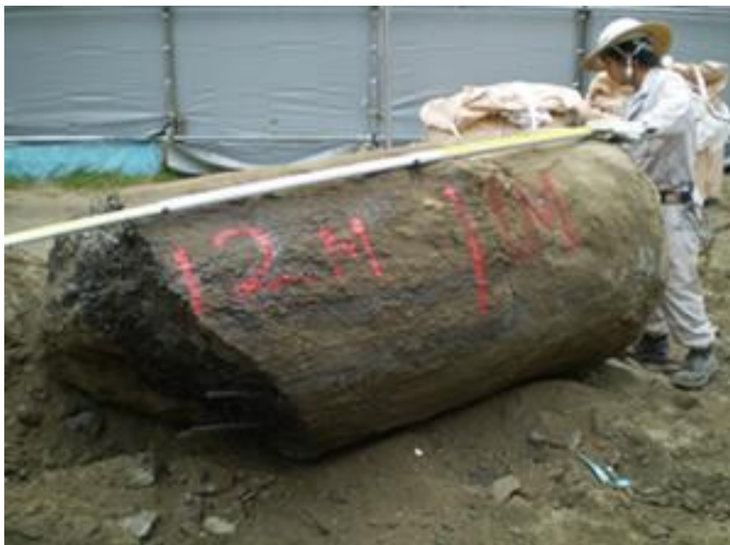
Underground obstacle removal situation(cast-in-place pile) (地中障害物撤去状況-場所打ち杭)
