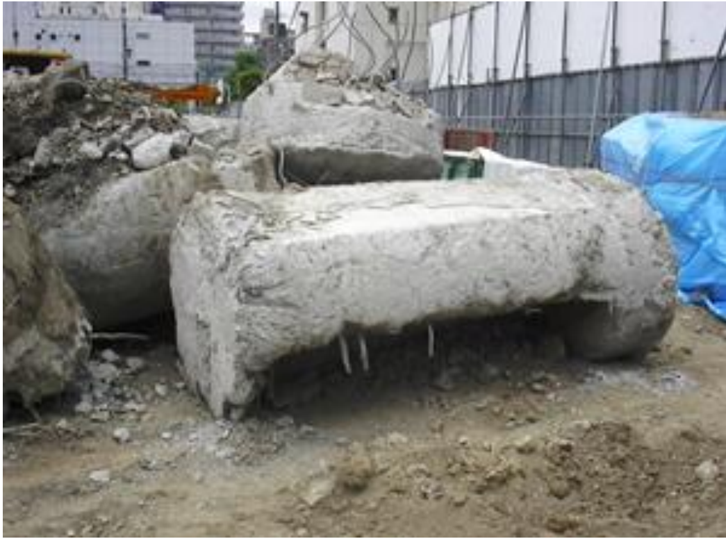
Underground obstacle removal situation (underground beam) (地中障害物撤去状況-地中梁)
