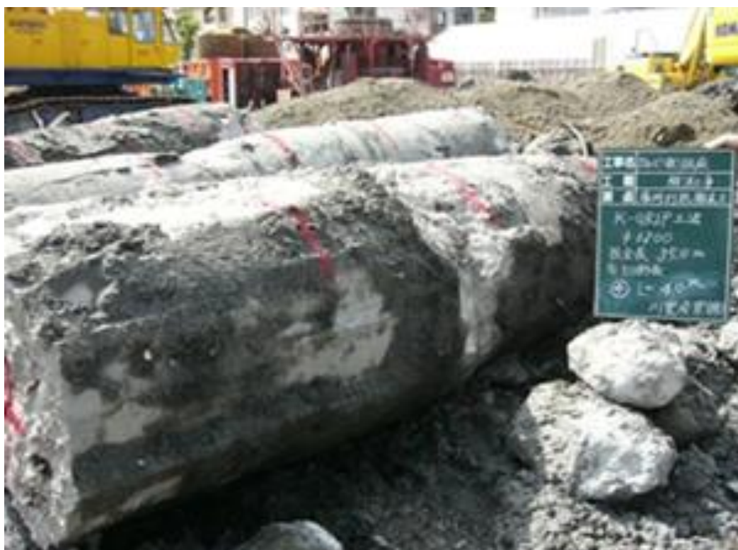
Underground obstacle removal situation(cast-in-place pile) (地中障害物撤去状況-場所打ち杭)
