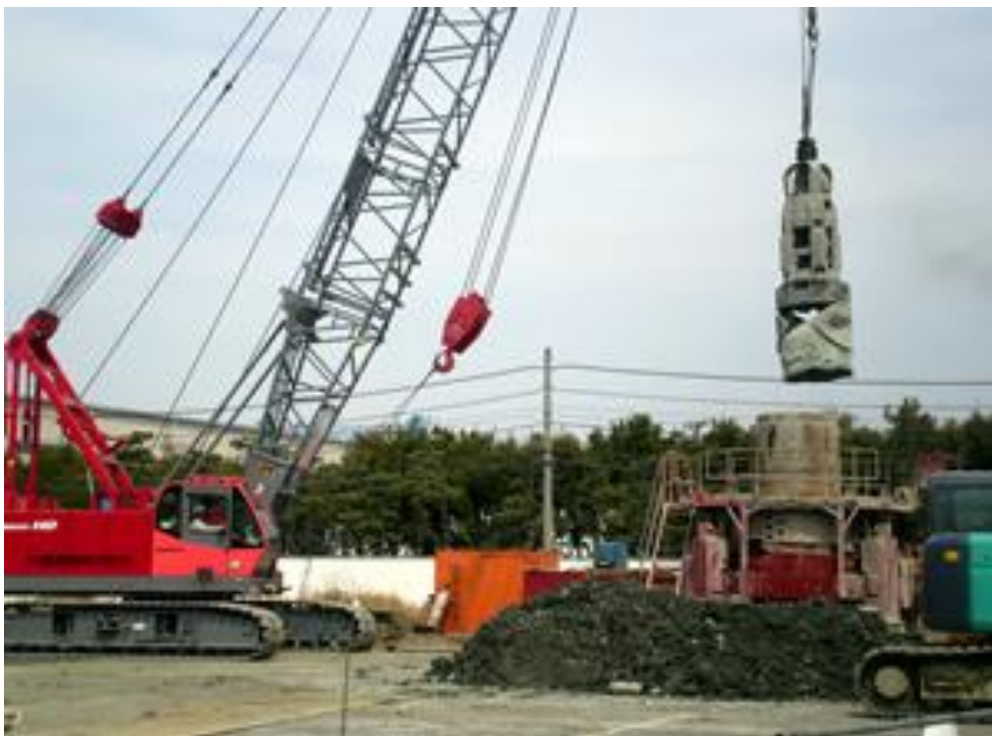
Underground obstacle removal situation (underground beam) (地中障害物撤去状況-地中梁)
